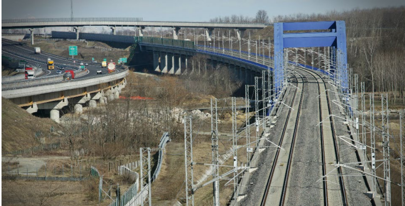
Client: C.A.V. TO-MI Description: Construction of infrastructures HS Railway Line To-Mi in Brandizzo - Agognate - Biandrate
