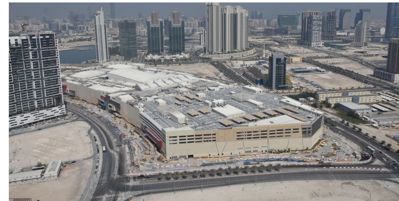
Client: AL FARWANIYA PROPERTY Description: Construction of the Abu Dhabi Reem Mall - UAE
