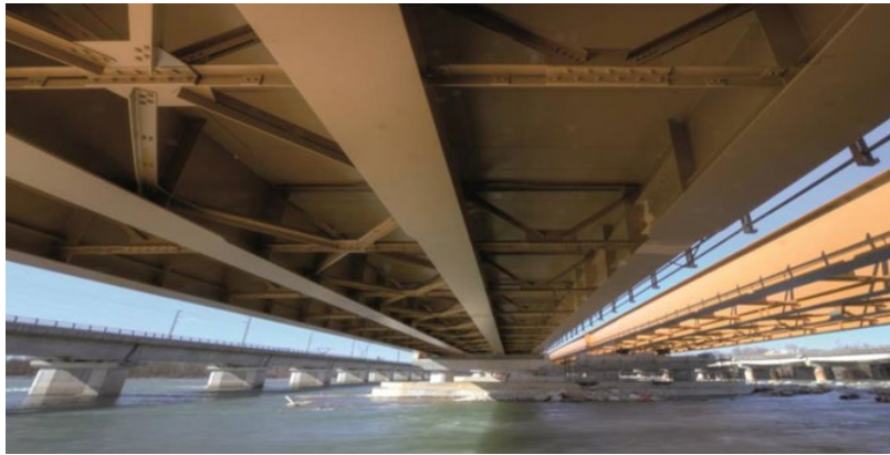
Client: S.A.T.A.P. S.p.A. Description: Rehabilitation and improvement works on A4 Highway, Bernate Bypass
