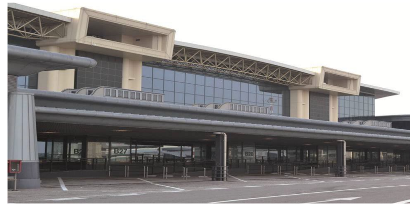
Client: S.E.A. S.p.A. Description: Construction Apron, service roads, terminal enlargement construction of ENAC Blg-Milano Malpensa Airport -Terminal 1
