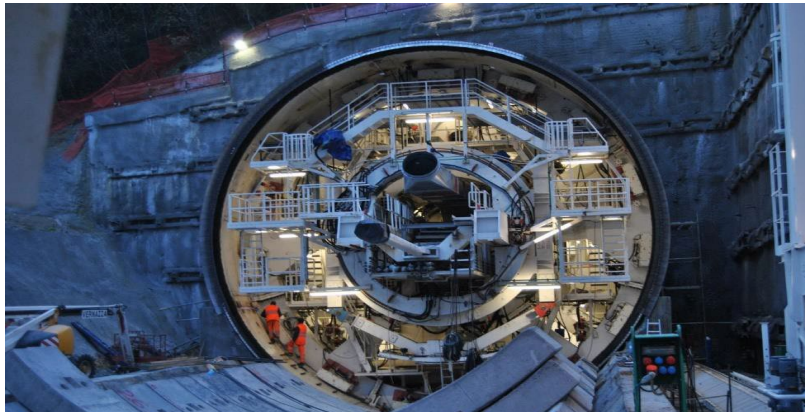
Client: ANAS S.p.A. Description: Construction of Bypass State Road S.S. 1 Aurelia - ALBISOLA (Savona)
