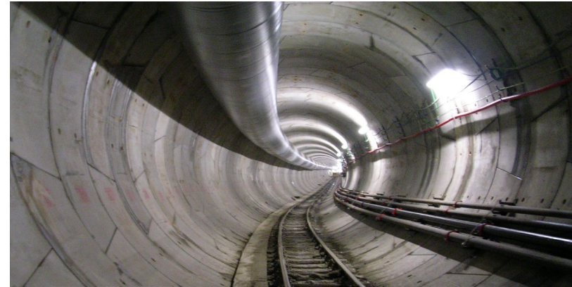
Client: M.N. Metropolitana di Napoli S.p.A. Description: Construction works Dante- Garibaldi route, Secondigliano warehouse and workshop, Piazza Dante station and Montesano corridor- Line 1
