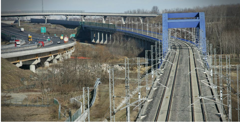
Client: C.A.V. TO-MI Description: Construction of infrastructures HS Railway Line To-Mi in Brandizzo - Agognate - Biandrate
